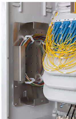
Fiber Distribution Hub MDP EL 432/864
